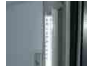
Illuminazione a led LED lighting
